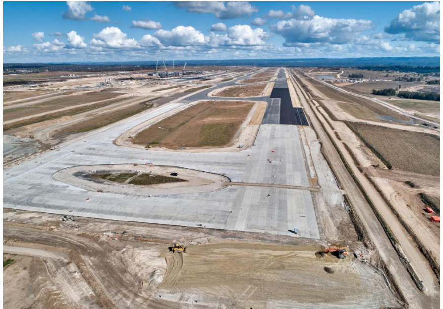
Aerial photo of the concrete pavement on the end of the runway, taken August 2023
